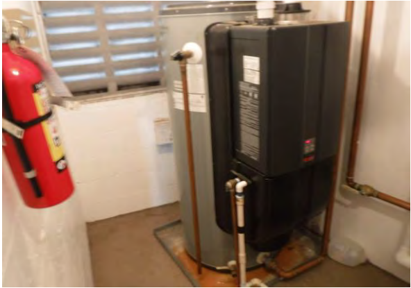
43 Water Heater #2 Overview
