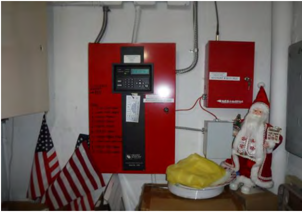
17 Fire Alarm System
