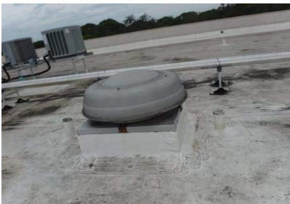
77 Power Roof Vents
