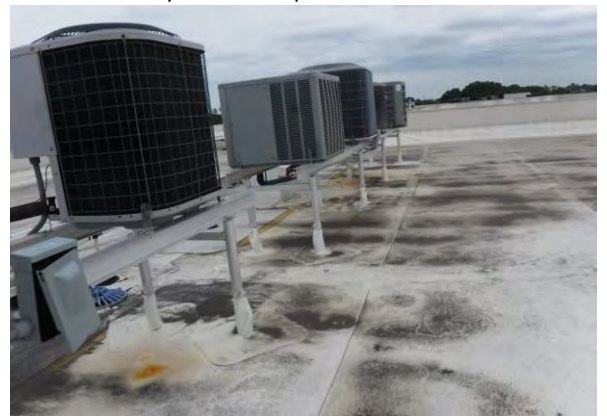
38 HVAC Stands on Roof
