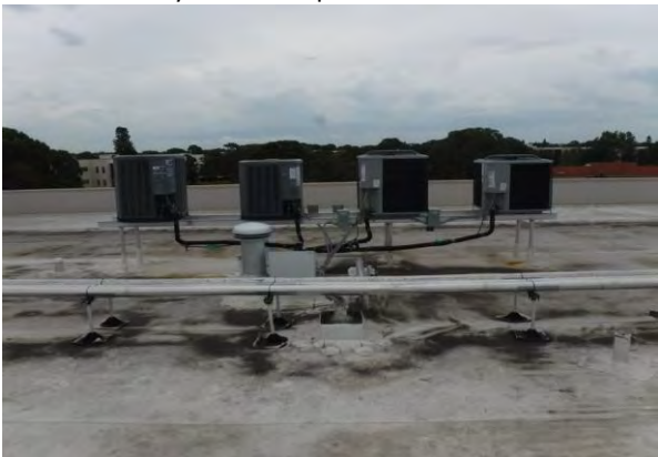
39 HVAC Stands on Roof
