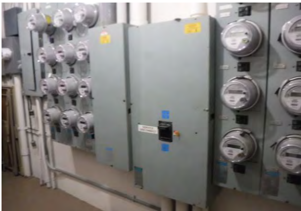
45 Main Electrical Panel/Disconnect
