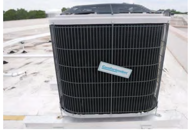
36 Laundry Room Compressor
