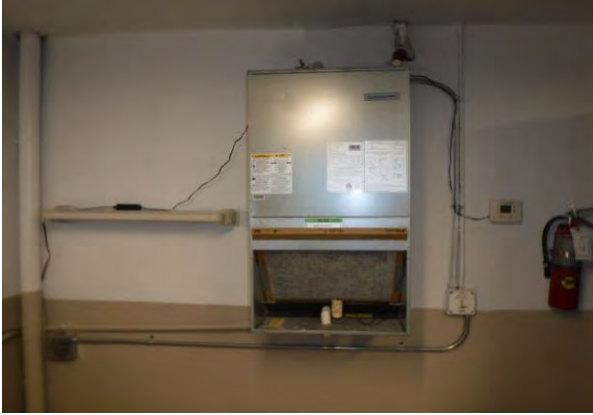
35 Air Handler in Laundry Room
