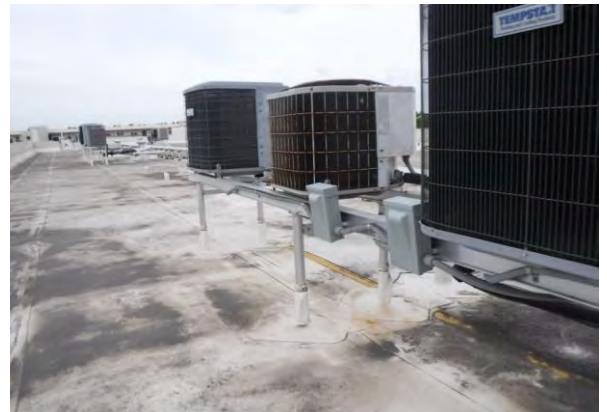
40 HVAC Stands on Roof
