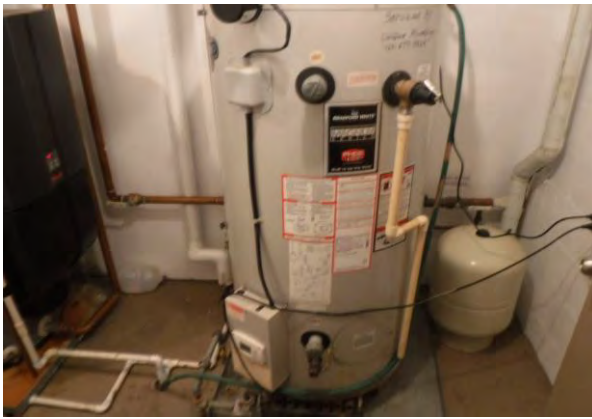
41 Water Heater #1 Overview
