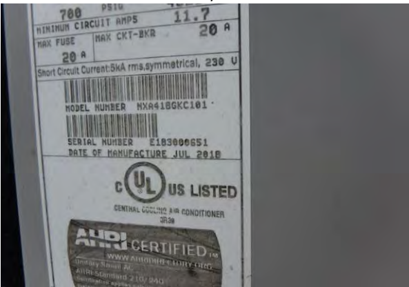
37 Laundry Room Compressor Data Plate
