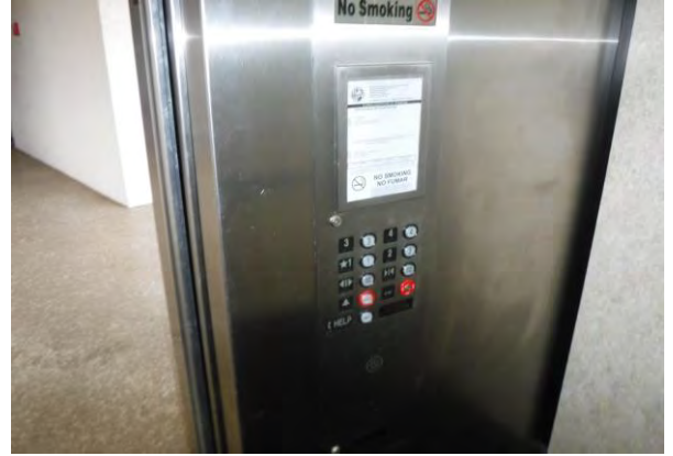
20 Elevator Cab Overview
