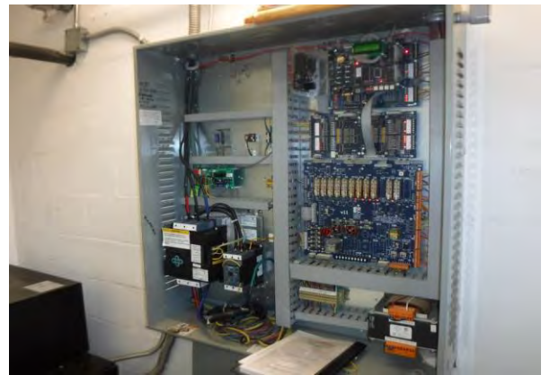
22 Elevator Motor and Controls
