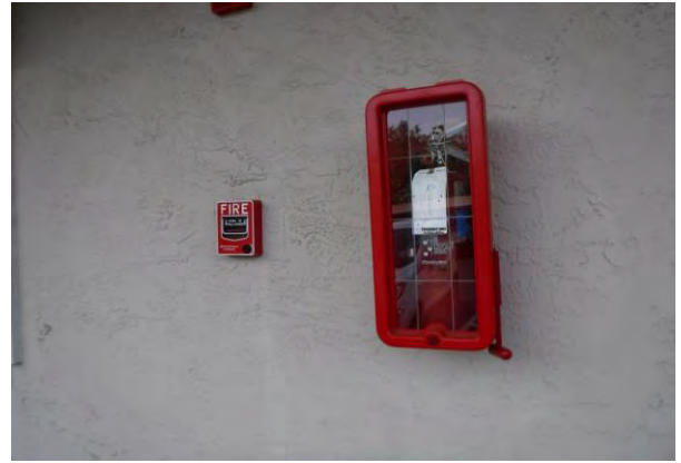
18 Fire Alarm System Pull Stations
